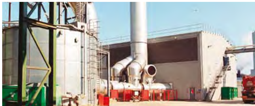
Two SGT-300 gas turbines provide Norbord with electricity and heat at their board manufacturing plant in Scotland, UK.
