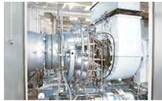
SGT-300 core engine test facility.
