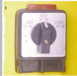
Voltage selector switch
