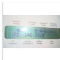
250KW GENERAC DIESEL GENERATOR...
