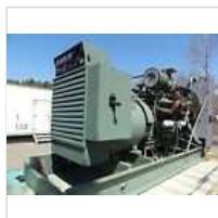
670 KW Generator 16V92 Detroit Diesel
