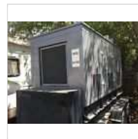
Generac Diesel 200KW 60Hz, 480V Mobile... $19,000.00
