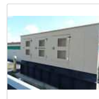
300 kW Generac Diesel Generator ~...
