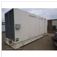
400 kW Diesel CAT Generator
