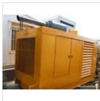
CATERPILLAR 265KW Generator 3 Phase...
