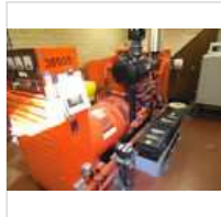
DMT-Cummins Generator Set 125 kW
