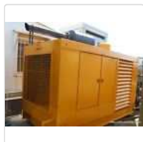
CATERPILLAR 265KW Generator 3 Phase...
