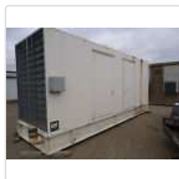
400 kW Diesel CAT Generator
