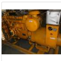
CATERPILLAR D333 DIESEL GENERATOR...
