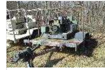
1989 Libby Corporation MEP 003A Generator Set
