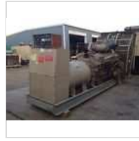
1987 Diesel 1200 KW Cummins Genset... $51,900.00
