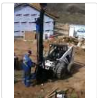
Deeprock Ram 10 Water Well Drilling rig...
