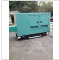
Cummins Diesel 35 KW Standby Generator
