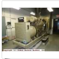
CUMMINS 500 KW DIESEL GENERATOR...
