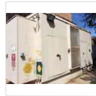
Caterpillar Diesel Generator 3508 DI...
