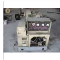
generator military libby welding compa...
