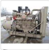
Cummins 400 KW Genset Backup Dies...
