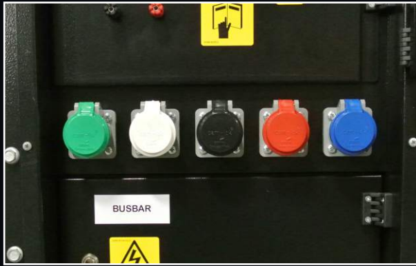
Camlocks are standard in addition to the lugs for easy color coded hookups when using distribution panels and boxes.
