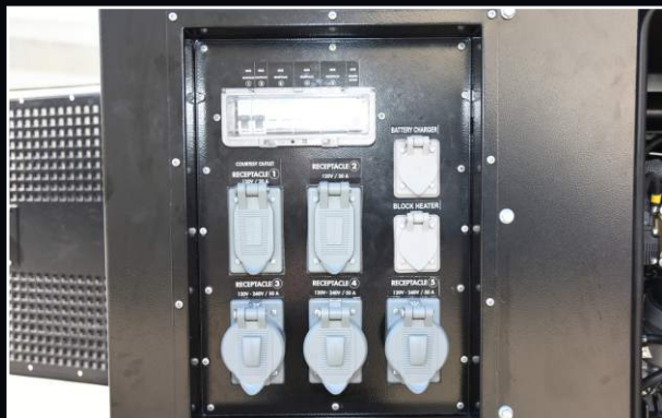
Courtesy outlets available in all phases at proper voltage.
