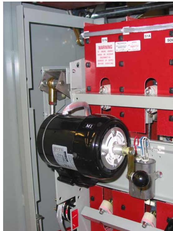
1000-3000A Transfer Switches
