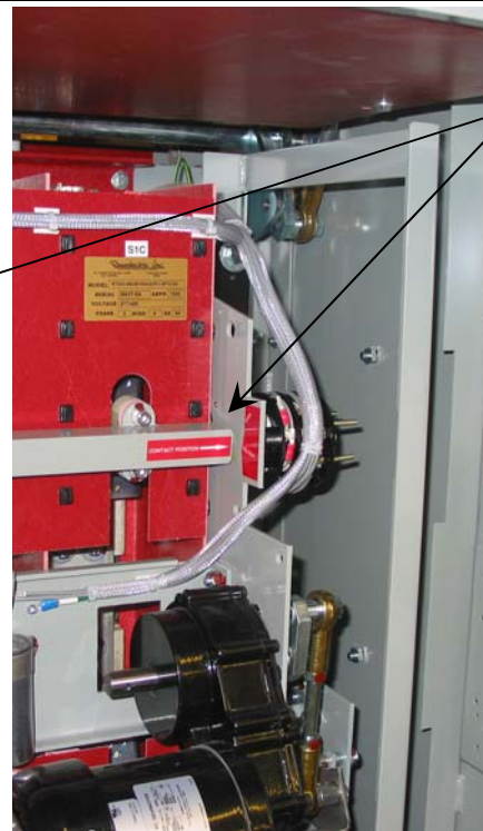
1000-3000A Transfer Switches
