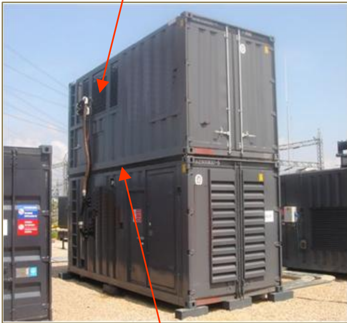
Gap between containers uses sealing strip to reduce noise levels
