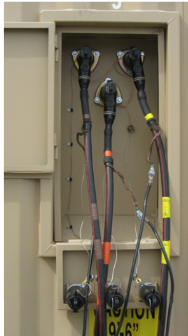
Load Connection Box (4160V)
