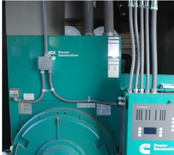
Genset Output (4160V)
