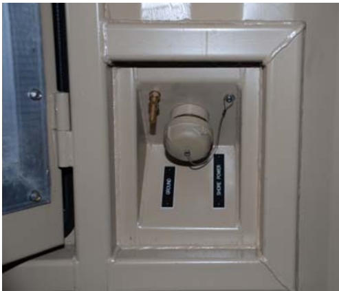
Shore Power Entrance
