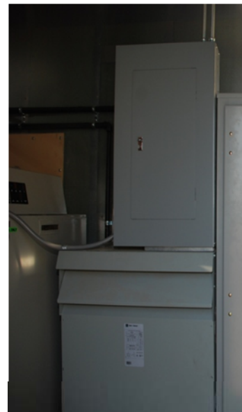
Transformer (4160V Primary/480V Secondary)
