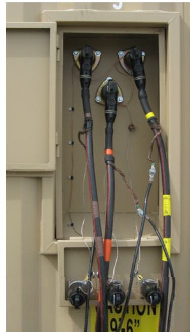
Load Connection Box
