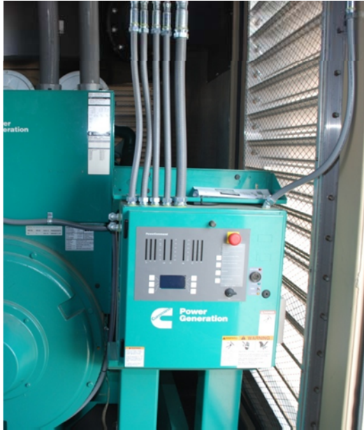
Generator Control Panel
