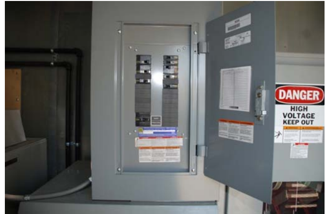
Shore Power Panel (120/208V 3 PH)
