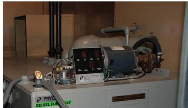
Daytank Pump & Controls (120V)
