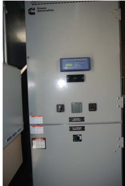
Breaker (4160V) – operator view
