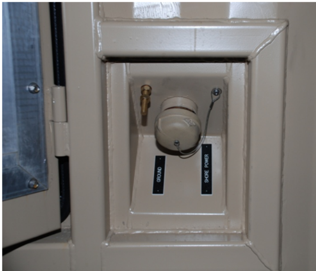
Shore Power Inlet
