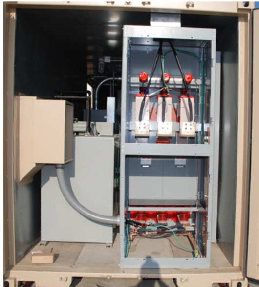
Breaker (4160V) – output view
